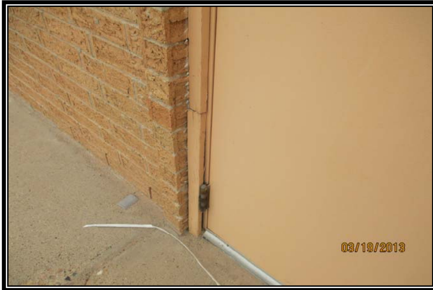
BRICK VENEER MOVEMENT / DAMAGE AROUND DOOR FRAME
