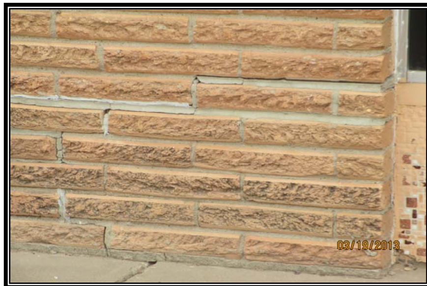
CRACKS IN EXTERIOR BRICK VENEER
