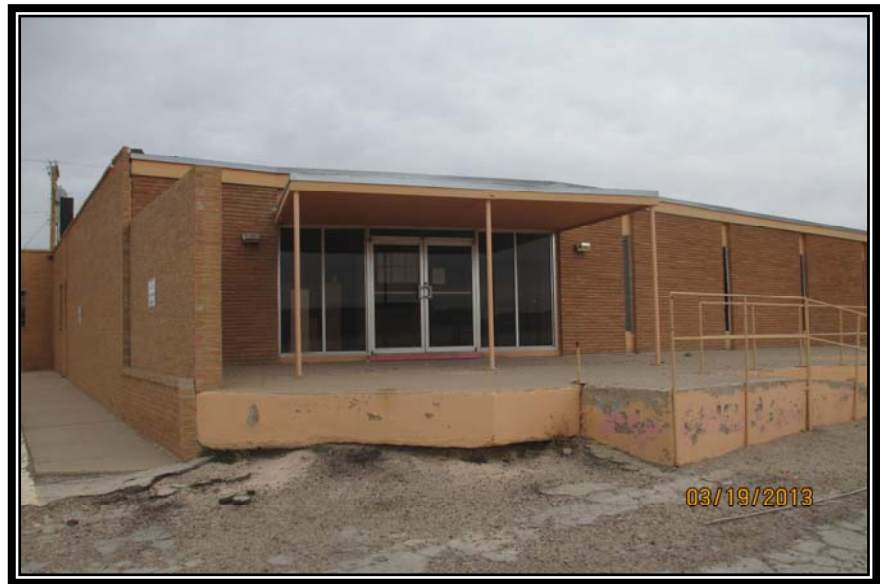
LOADING DOCK – NOTE POOR CONDITION OF PAVING / ACCESS TO THE LOADING DOCK
