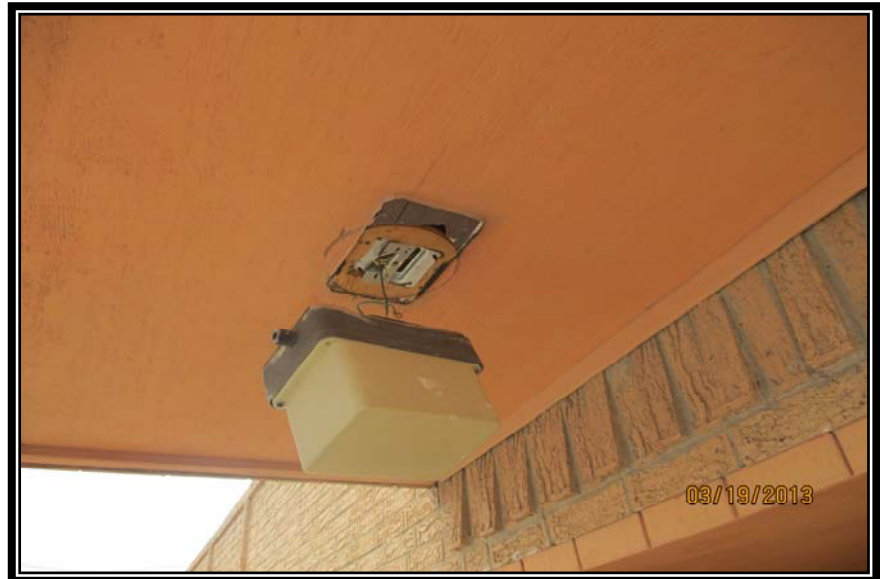
SECURITY LIGHT DAMAGE IN PORCH ABOVE FRONT ENTRY
