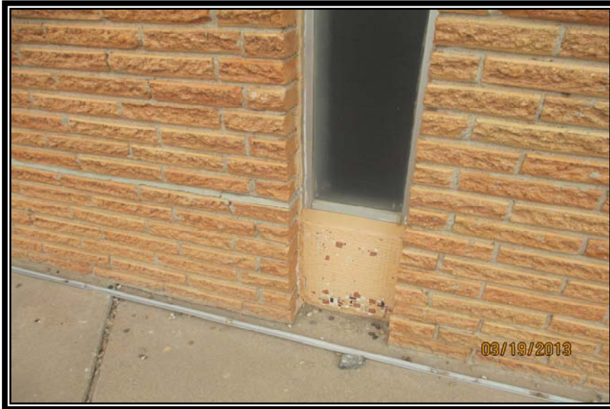
DAMAGE TO TILE BELOW WINDOW
