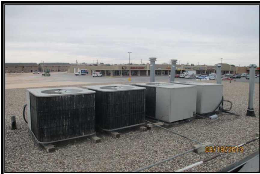
VIEW OF ROOF AND HVAC UNITS LOOKING SOUTHWEST – NOTE HVAC UNIT DAMAGE
