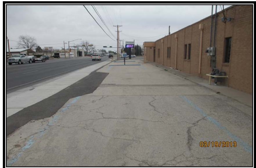
LOOKING EAST AT FRONT OF HANDICAP PARKING AREA – NOTE POOR CONDITION OF PAVING
