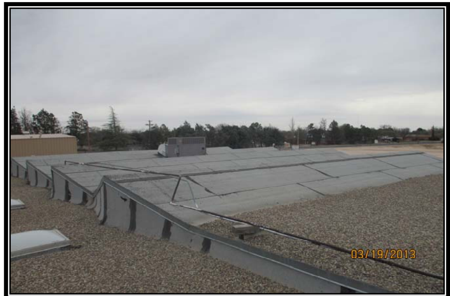
VIEW OF PITCHED ROOF AND HVAC UNIT IN SOUTHEAST CORNER OF BUILDING
