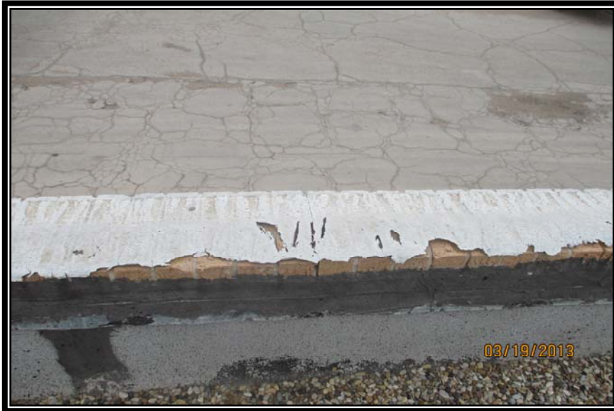
DAMAGE TO TOP OF PARAPET WALL
