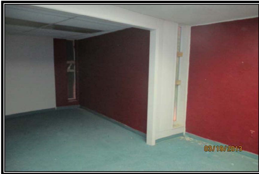
TYPICAL OFFICE ON SOUTHEAST CORNER OF BUILDING – NOTE IRREGULAR WALL AND CARPET DAMAGE
