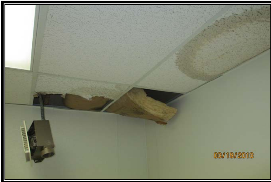
CEILING DAMAGE IN RESTROOM
