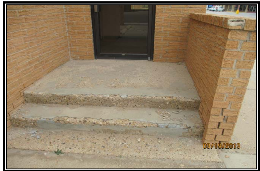
DAMAGE TO STEPS AND BRICK WALL AT WEST ENTRY VESTIBULE
