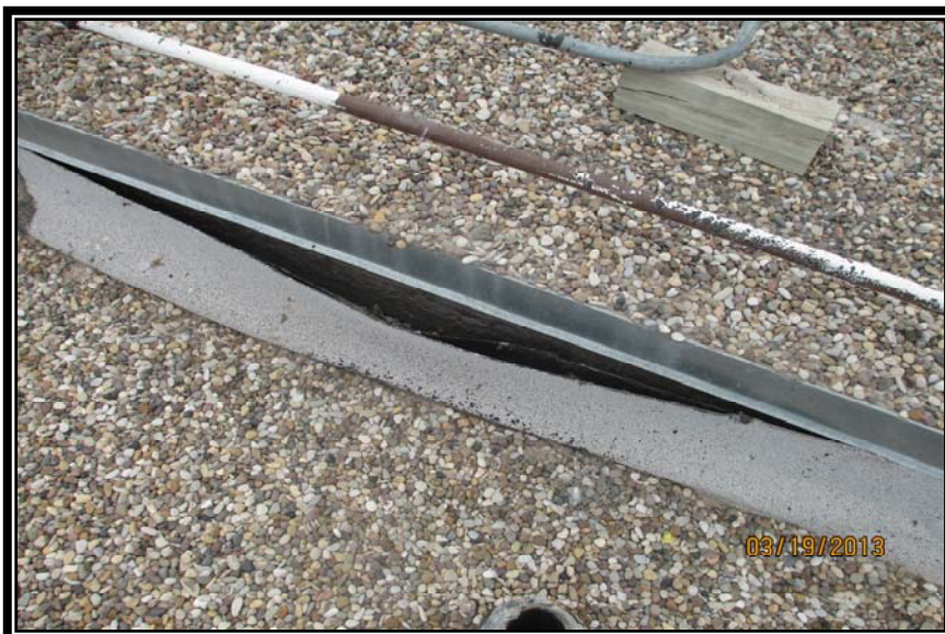
DAMAGE TO TAR AND GRAVEL ROOF
